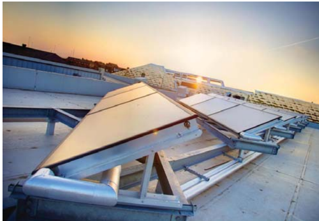
Solar water collectors mounted on roof
